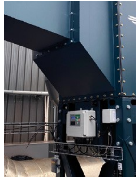
The ACDC (Camfil APC Advanced Control) control panel is designed to act as the intelligent centerpiece of the dust collection system.
